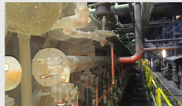
Original furnace burner and fuel train system before upgrades
