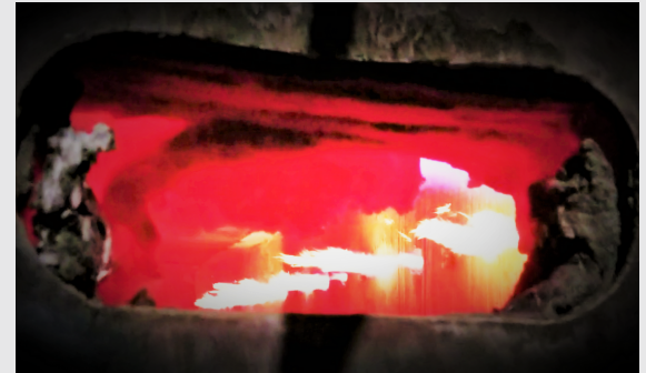
Flames in the furnace from the new burner system
